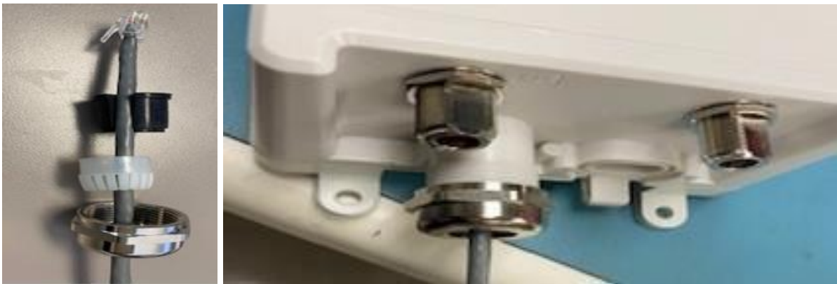
Figure 10: KONA Enterprise Gateway Module Cable Gland
